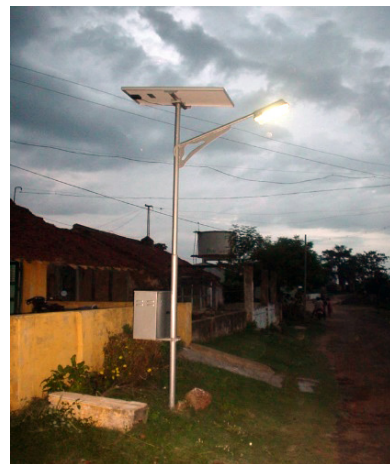
Figure 9: Solar street light
