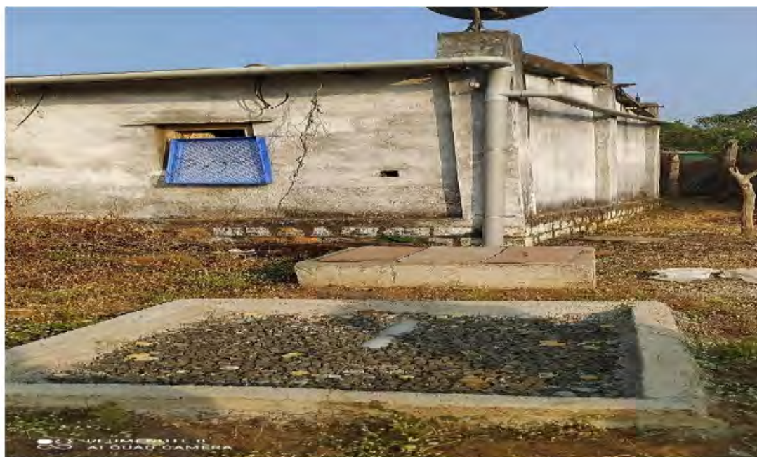
Roof top rain water harvesting structure
