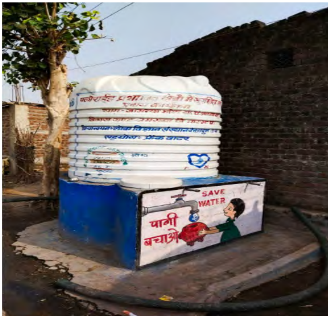
Water tanks installed in the community
