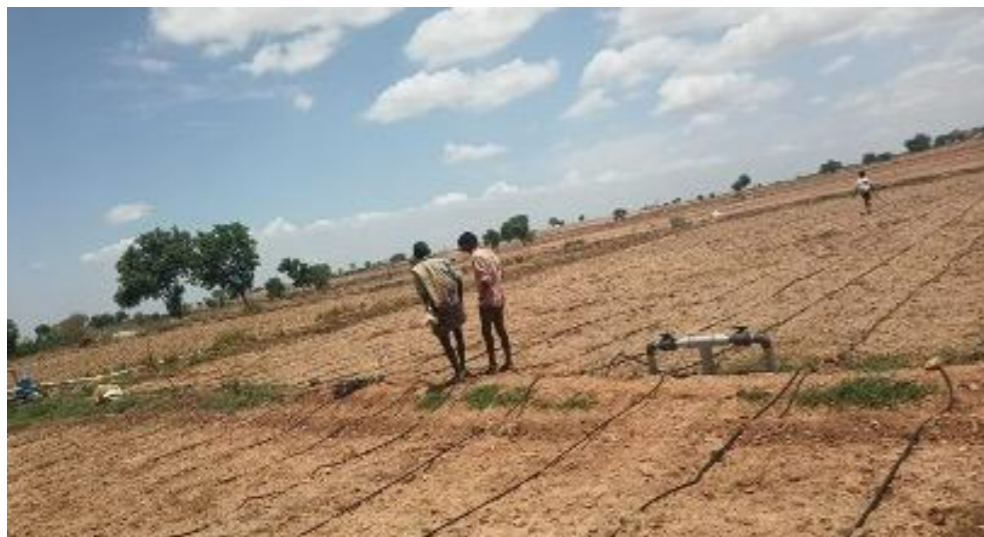
Photo of Drip irrigation system installed in a farmer's land
